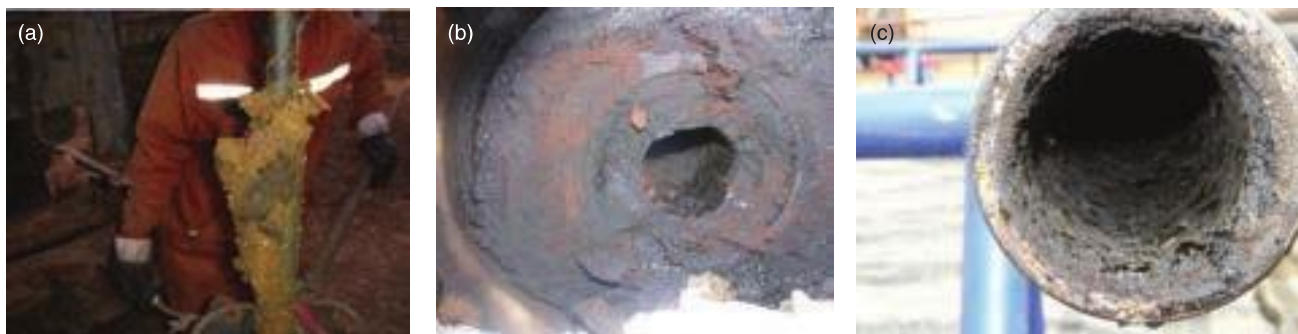
Fig. 1—The effect of wax deposition is shown on (a) a well tubing string, (b) a cross-section of a flowline, and (c) the inside of a tubular. Photos courtesy of Diversitech.
